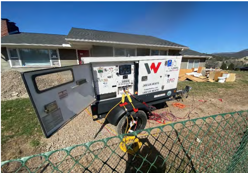
View of a portable generator utilized during the asbestos abatement at 137 Howard Street. View to the west.
