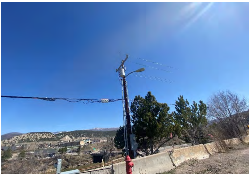
View of a pole-mounted transformer at the northeast corner of the property. View to the northeast.
